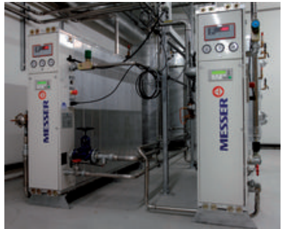
On site PSA Anlage
